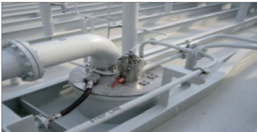
Example of a Framo hydraulic deepwell pump at deck level
