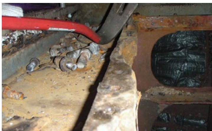
Heavy local corrosion of the flange of a box cooler.
