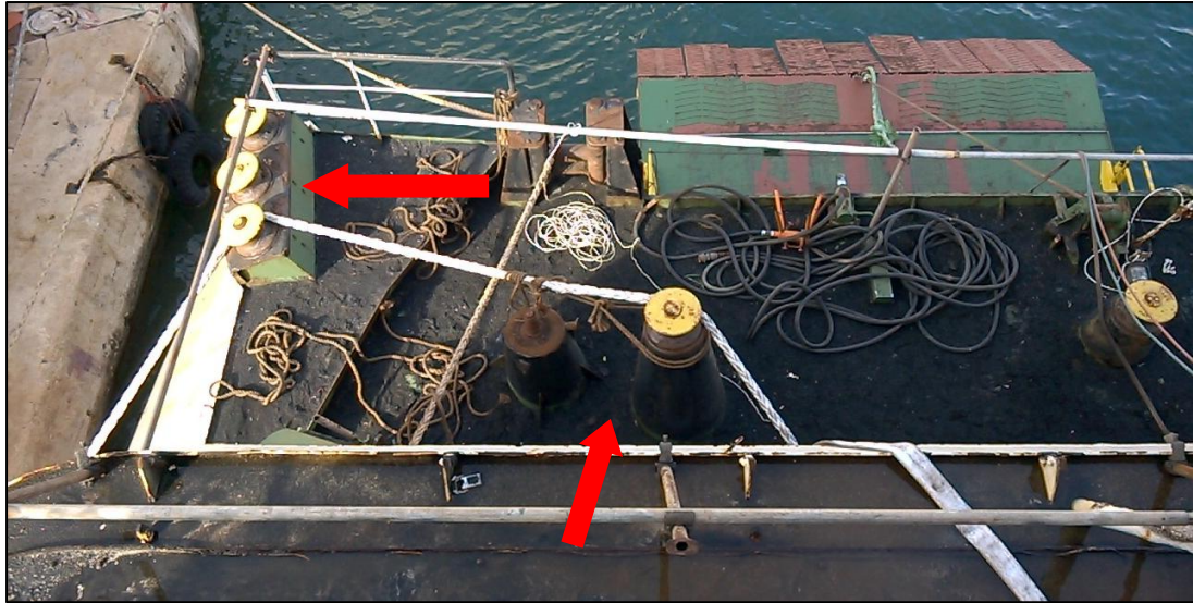
Figure 3: Open button-roller chock and pedestal fairleads on the aft mooring deck
