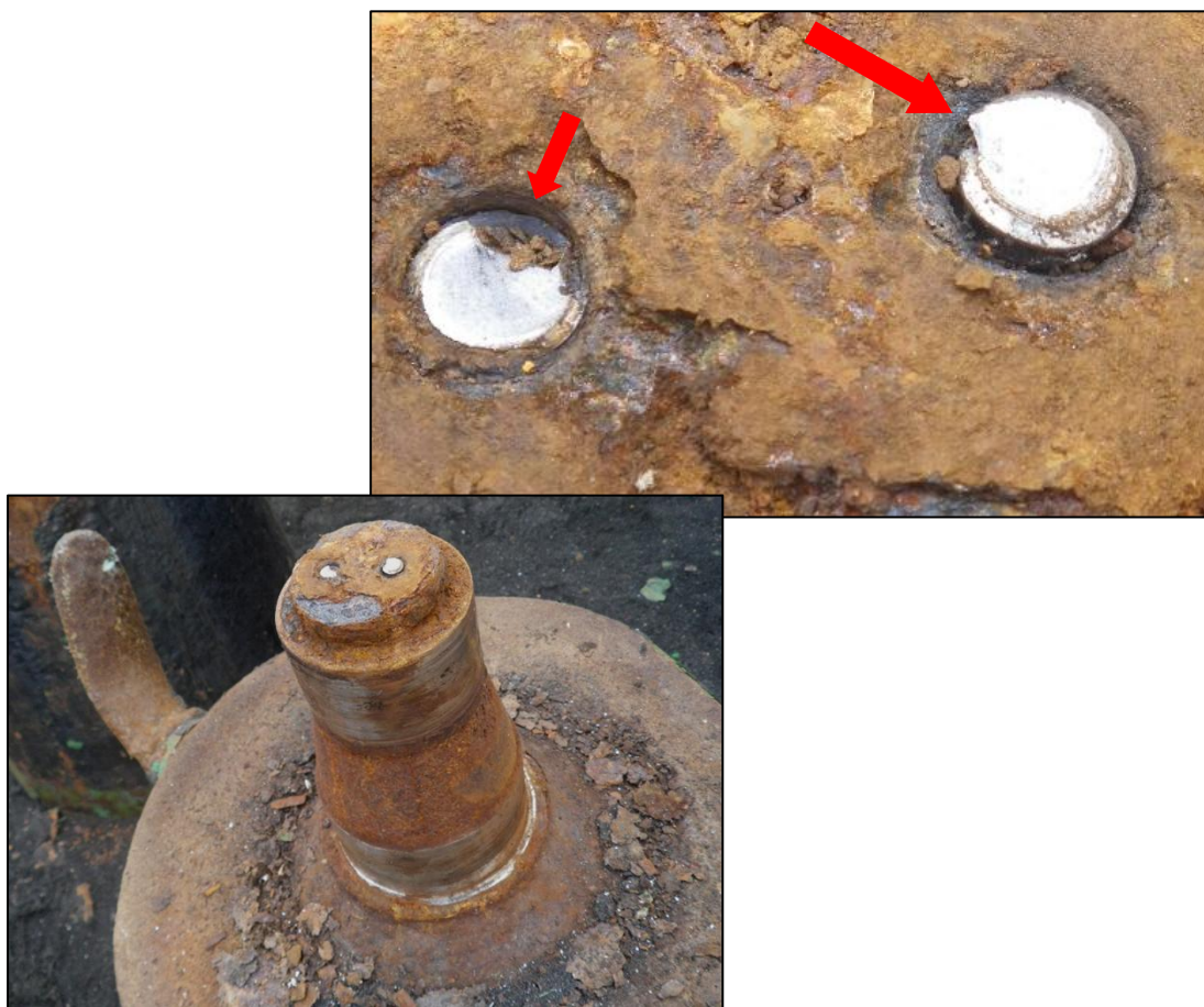
Figure 11: Details of the sheared bolts holding the roller-keep
