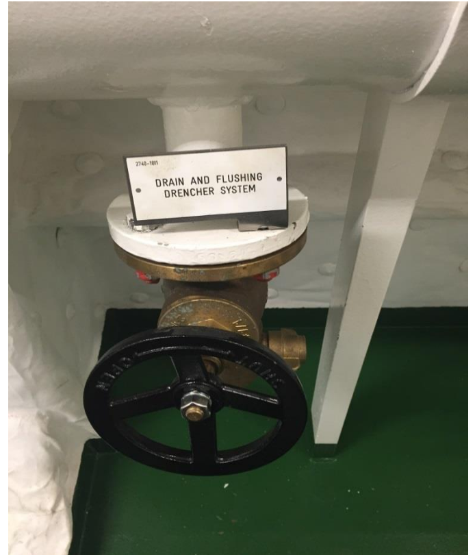
Fig 7: Drenching system flushing valve
