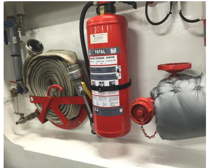
Fig 13: Portable fire-fighting equipment
