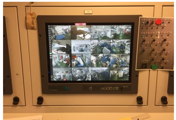
Fig 4: CCTV remote monitoring
