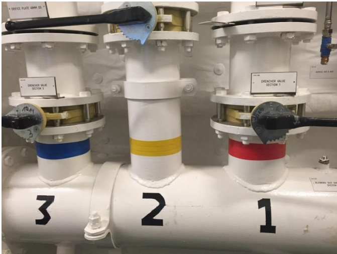
Fig 11: Drencher system valve labelling (colour coded)
