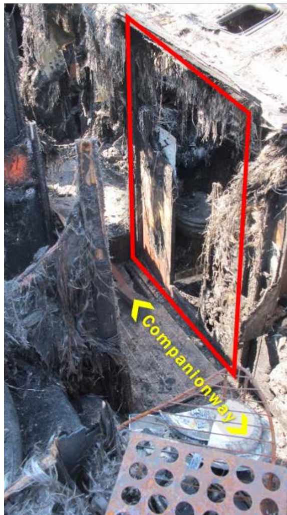
Lavatory where fire likely originated next to portside companionway between guest staterooms while looking aft to stateroom.
