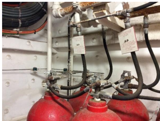
Image - Common arrangement of pilot bottles connected to system with flexible pipes
