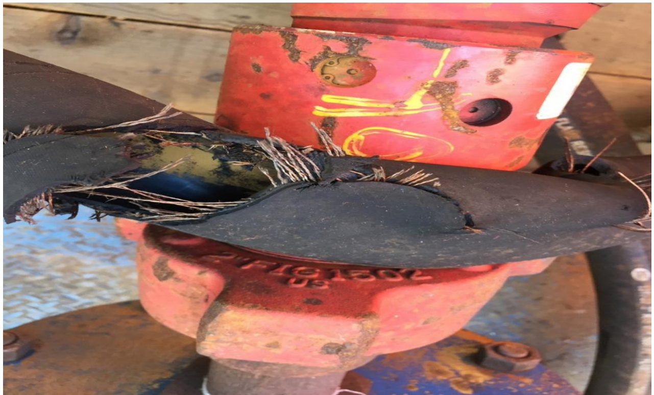
Photo 4: Faulty pre-commissioning system hoses
