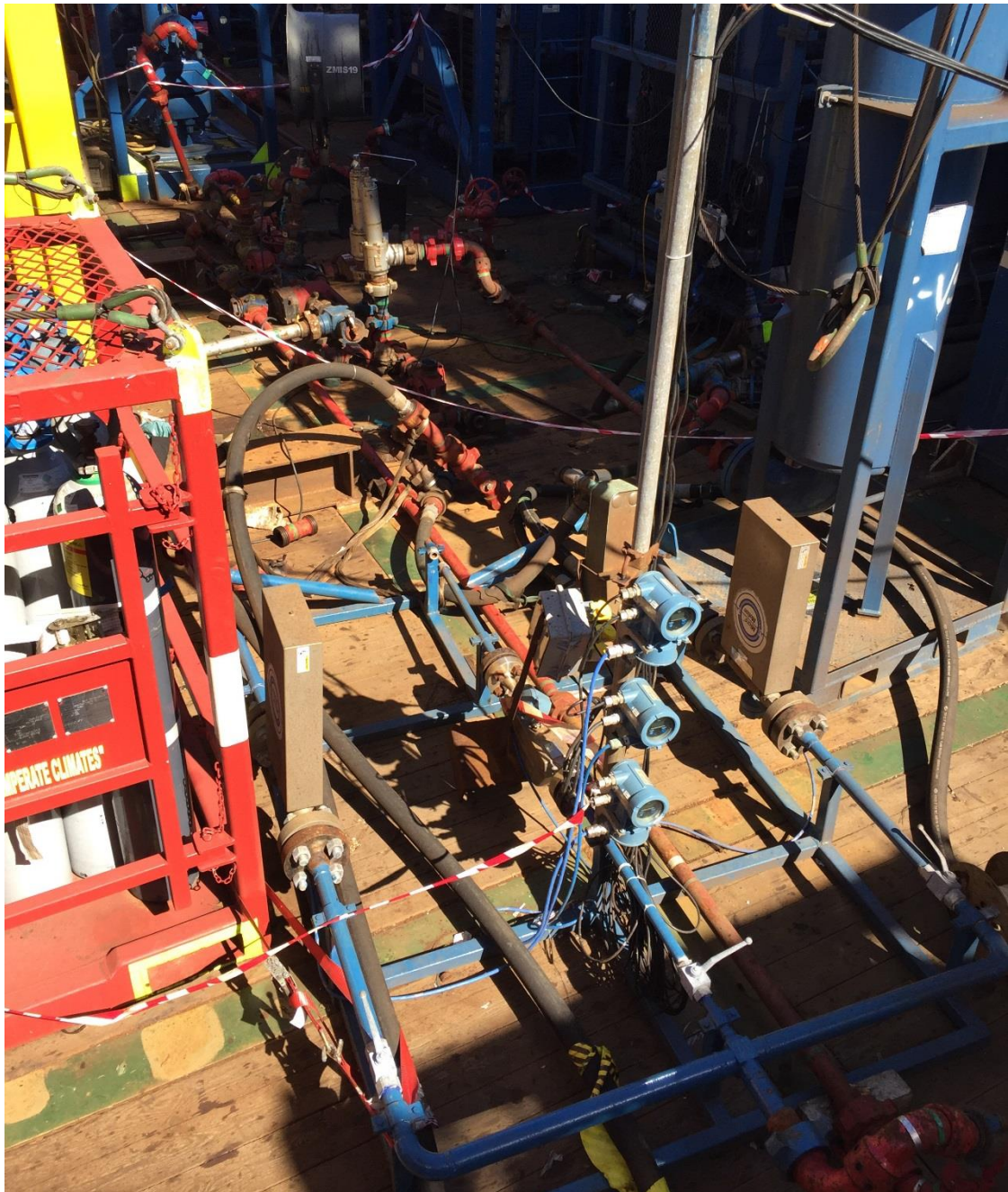
Figure 4: Pipes, hoses and valves placed between components on the open deck. Photo: The Brazilian Navy
