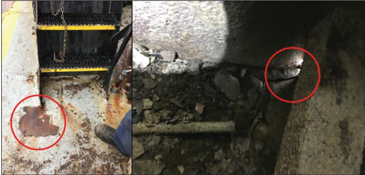
Pre-existing damage on the Tom Bussler . Left: severely corroded deck on the bow inboard of the port towknee. Right: corroded hole in the hull from within the bow void.
