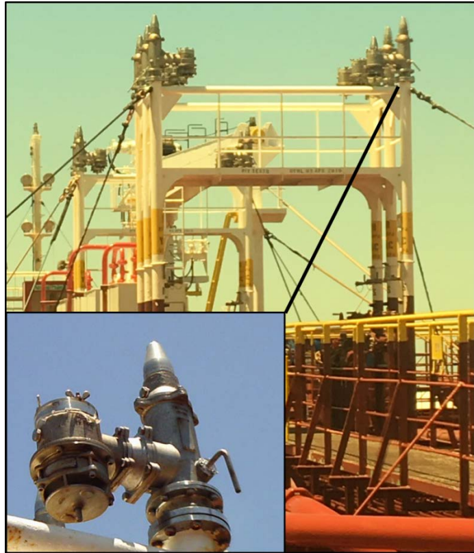
Pressure/Vacuum valves on board the main deck of the Fairchem Filly .
