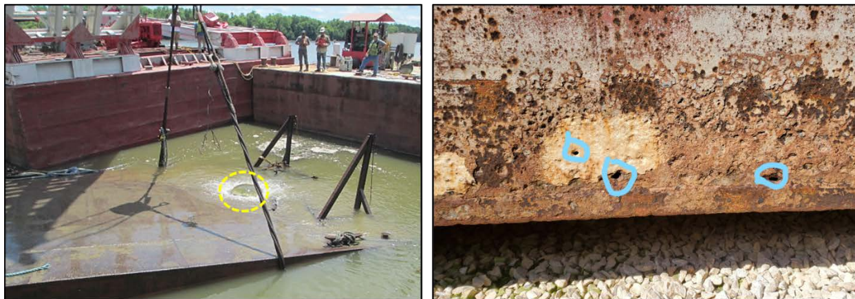
At left, water bubbles from the manhole on the top deck of the barge during salvage. At right, an annotated photo from the vessel company identifies holes on the side shell of the barge near the bottom plating. (Source: Coast Guard and Hex Stone)
