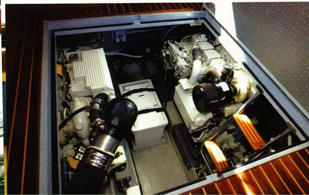
below There is a huge engine hatchway, and useful steps down have thoughtfully been provided.
