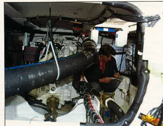
Below: the engineroom can be entered via the lazaret or a hatch in the saloon sole. There was ample room to move around and between our test boat's Cummins diesels.
