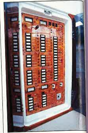
Above: set in the forward bulkhead near the helm position is a very comprehensive electrics panel. Below: twin 420hp Caterpillars were installed in our test boat.
