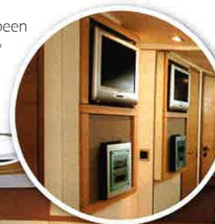
TV panel for the master cabin
