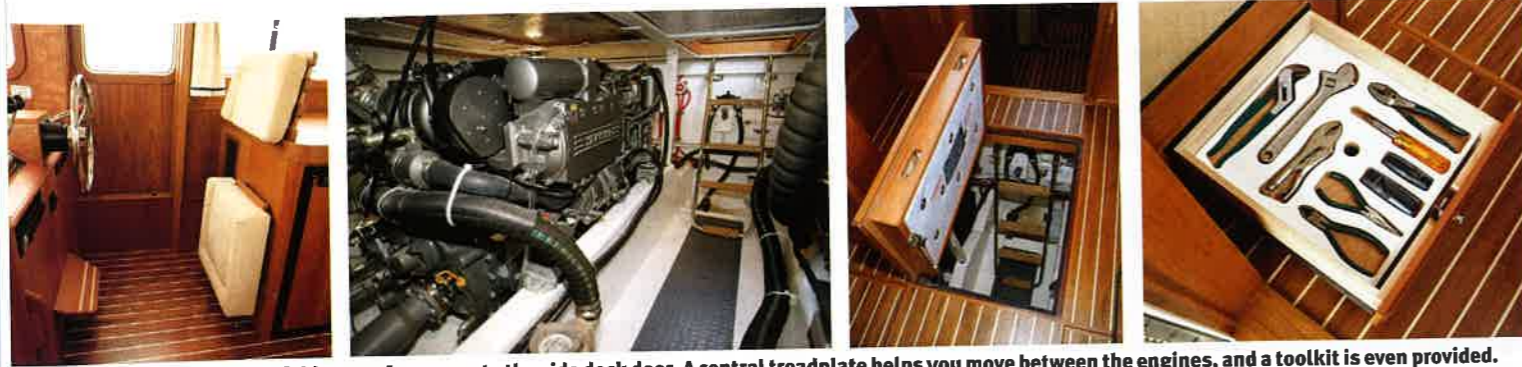
above The helm seat folds away for access to the side deck door. A central treadplate helps you move between the engines, and a toolkit is even provided.
