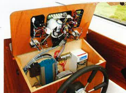
above ...with a lid giving easy access to the wiring.
