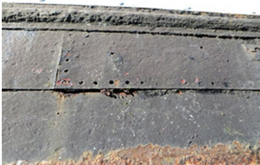
Photograph 1 Shear Strake Plate blown off the Side by Crevice/Jacking Corrosion on the Landing Strake Seam
