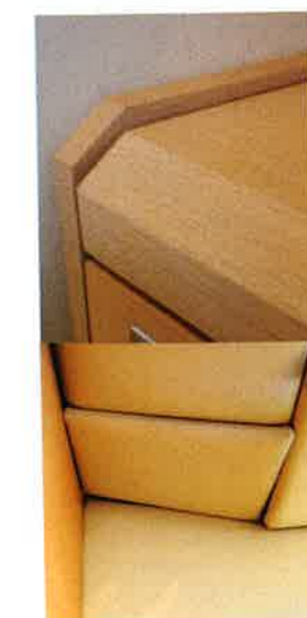
Poor finish dotted the 44's interior as with the disjointed cabinetry (top pic) and scruffy linings
