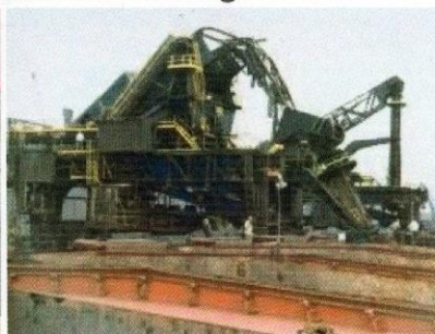
Catastrophic structural failure
